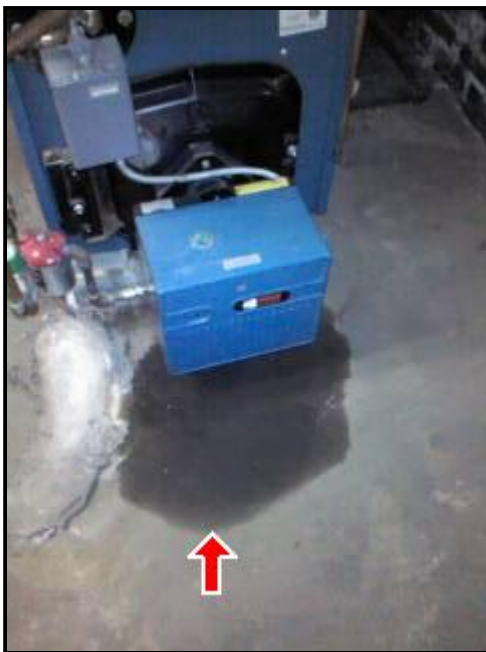
8.0 Picture 1 oil leak
