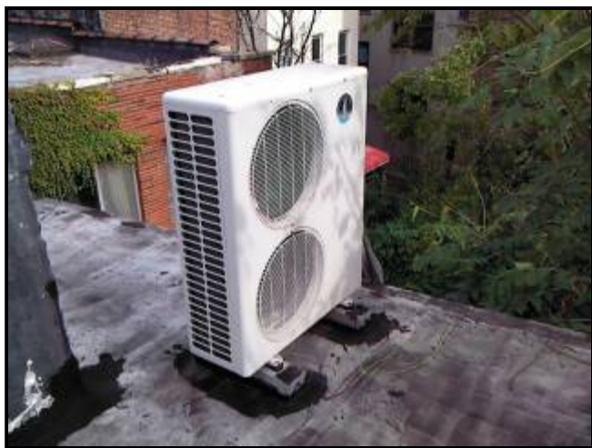
7.9 Picture 1 ductless AC unit, compressor
