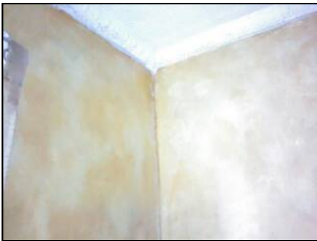
3.1 Picture 3 Water damaged wall in master bedroom
