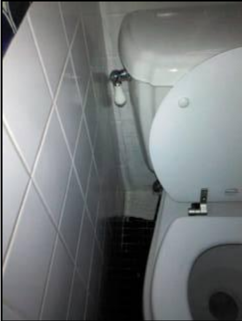
3.1 Picture 1 missing tiles
