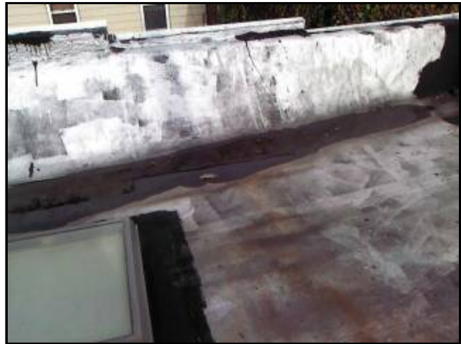
1.0 Picture 2 water not draining
