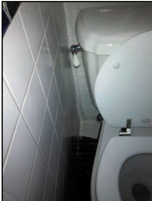
3.1 Picture 1 missing tiles
