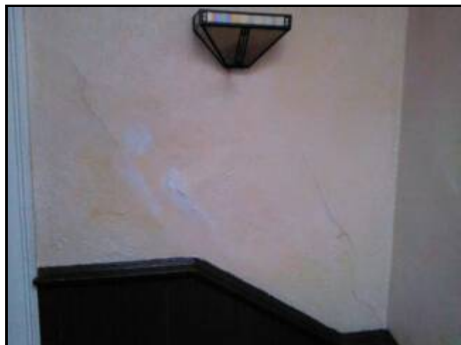
3.1 Picture 2 Wall cracks
