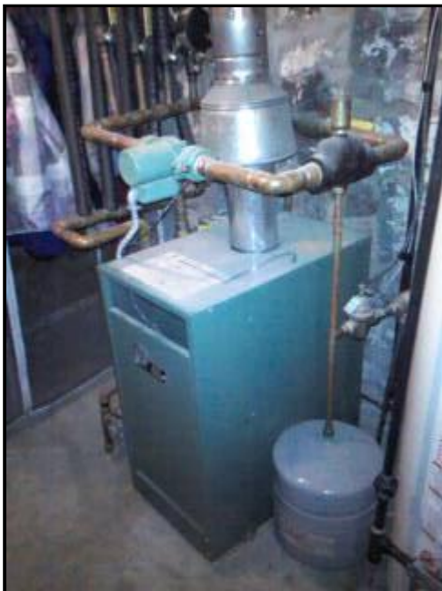
7.0 Picture 1 hot water boiler
