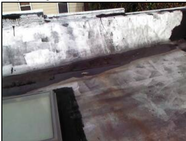
1.0 Picture 2 water not draining
