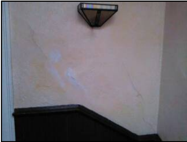
3.1 Picture 2 Wall cracks
